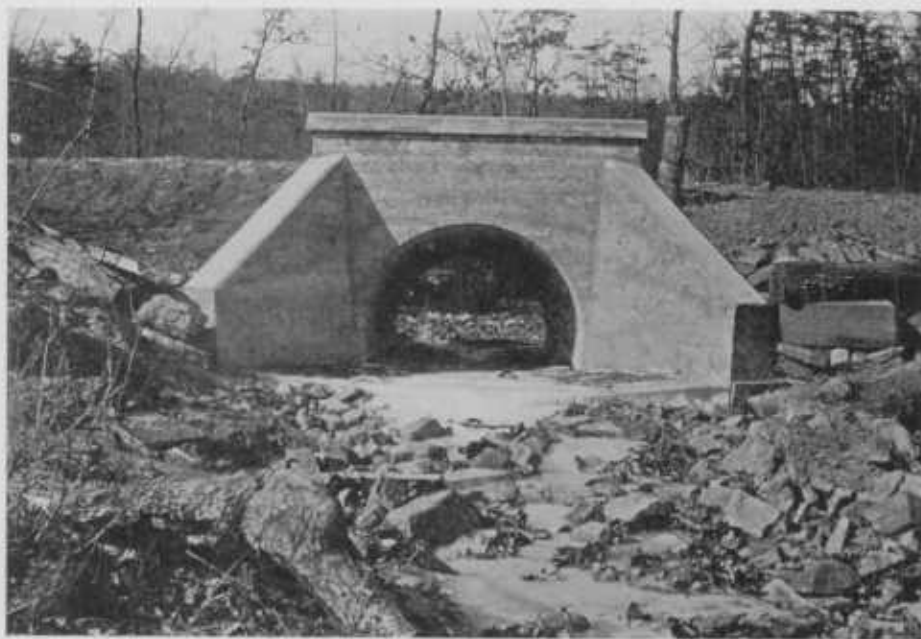
FIG. 2.—IMPROVED CULVERT ON RIVER ROAD BETWEEN CUMBERLAND AND CRESAPTOWN, ALLEGANY COUNTY, BUILT BY COUNTY ROADS ENGINEER.
