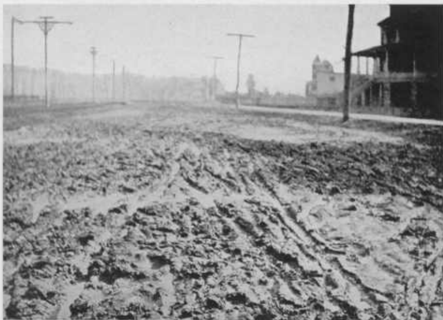
FIG. 1.—SECTION OF GWYNN OAK AVE., BALTIMORE COUNTY, BEFORE IMPROVEMENT.
